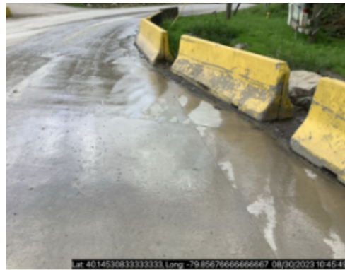
Industrial wastewater from the truck wheel wash, draining into the storm water dish
