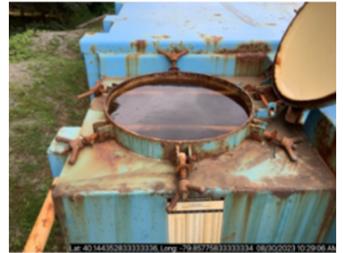
Fracking tank at leachate load-out completely full
