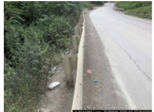
Mud and debris along Tyrol Blvd near Jonson Ave.
