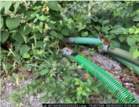
Hoses from the leachate positioned into stormwater ditch.
